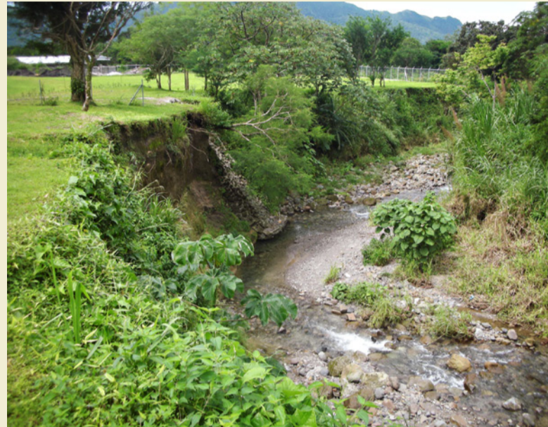
Los Portales, Rio Guayabo (Pre-Envirogrid Retaining Wall and Slope Protection System)
