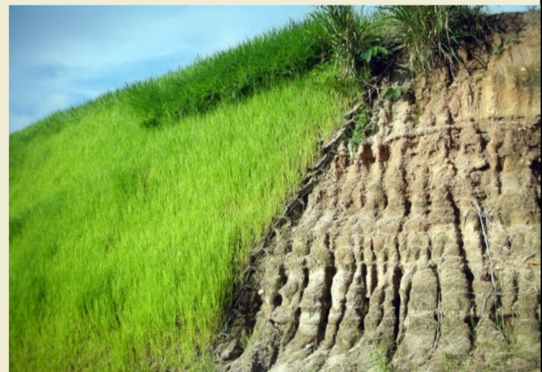
Finished Project showing termination of material (Left is complete, Right is original slope)
